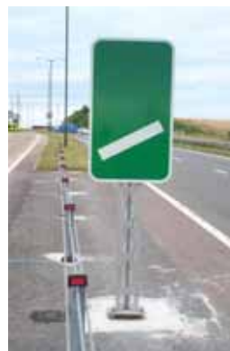
Lattix Crash Absorbent Posts and Wire Rope Safety Fencing
